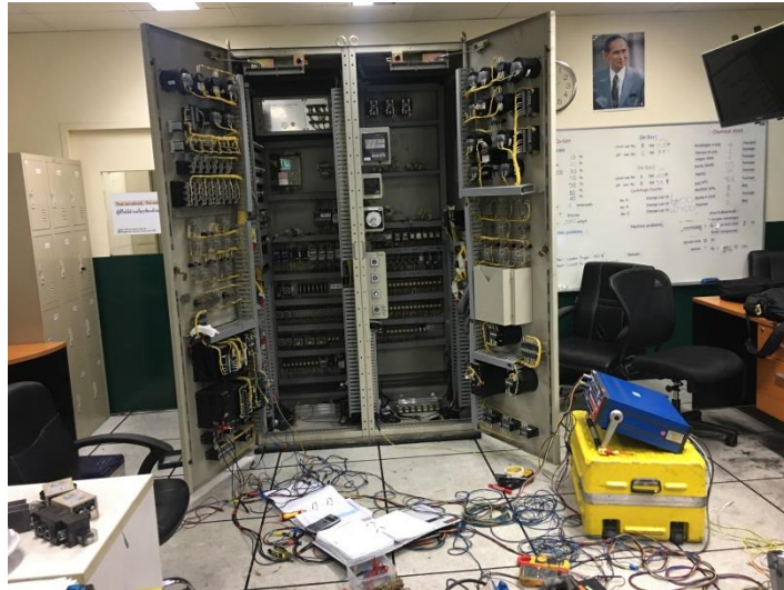
រូបទី ៩ រូបថត GCP Panel - Protective relay , metering, control device test
