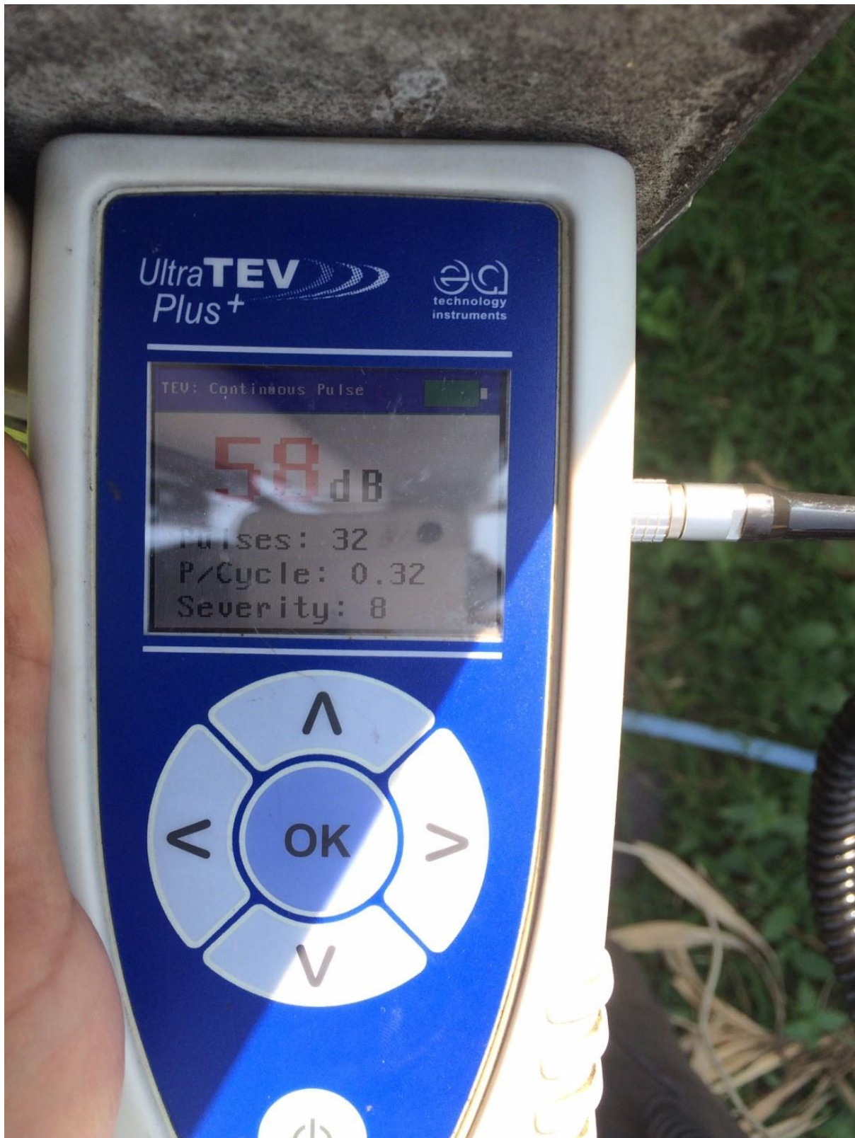
PD TEST BY TEV MODE AT 22 kV DISTRIBUTION POLE METERING
